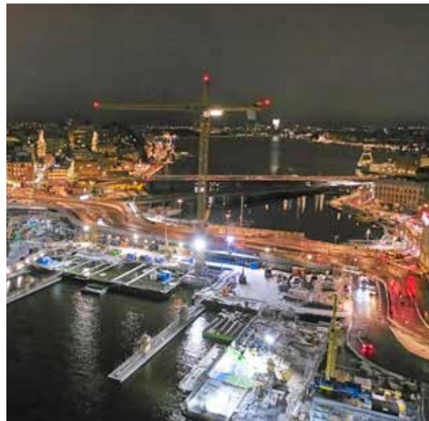
There is a stretch of about 500 metres of SoundGuard, the shell protection for both work zones and road users, that runs from the Gamla stan metro station to Kornhamnstorg.
