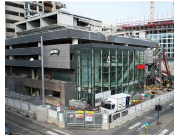
Construction projects in central Oslo, where the buildings are protected using GP Link and SoundGuard.
